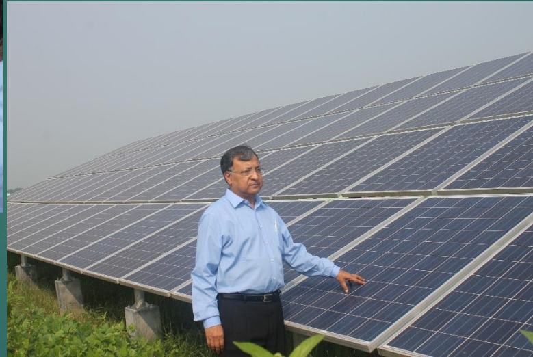
Solar PV for Irrigation pump
