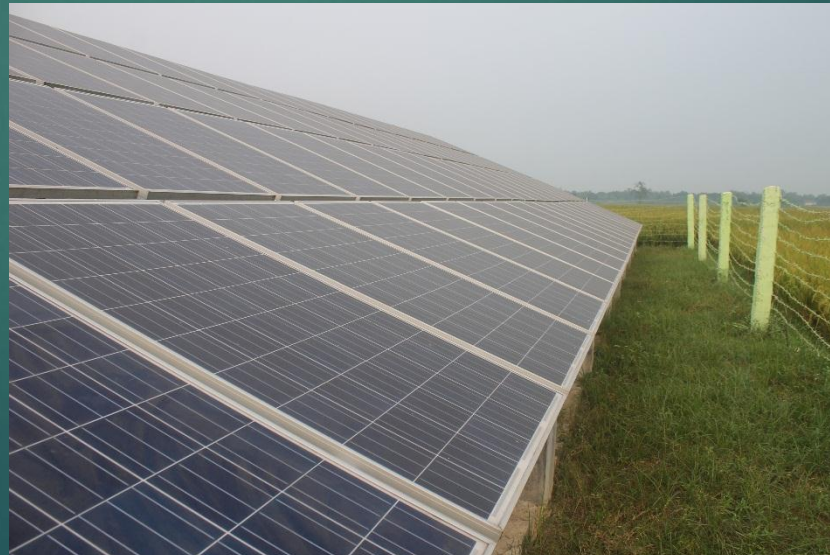
Solar PV installed for irrigation pump
